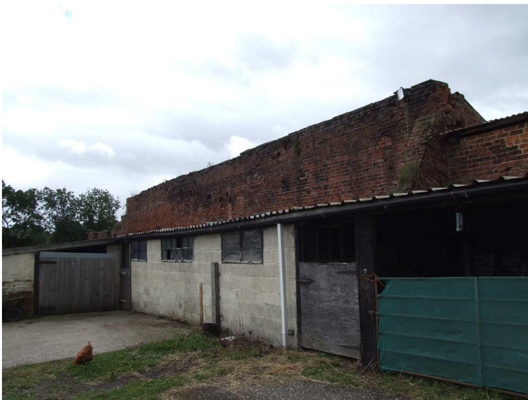
July 2010 – Remaining evidence of Spa Mill. Brick built wall once thought to be 4 storeys
